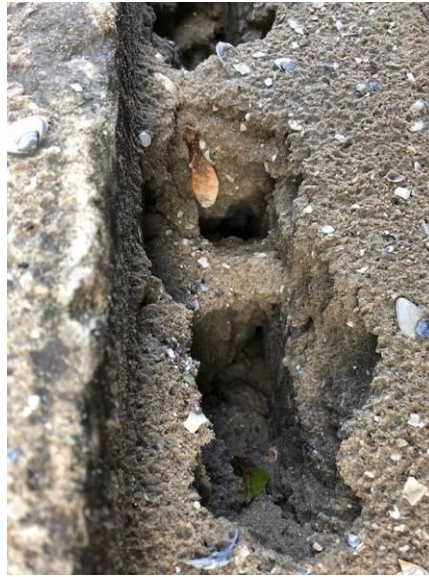
De gaten in close-up.
